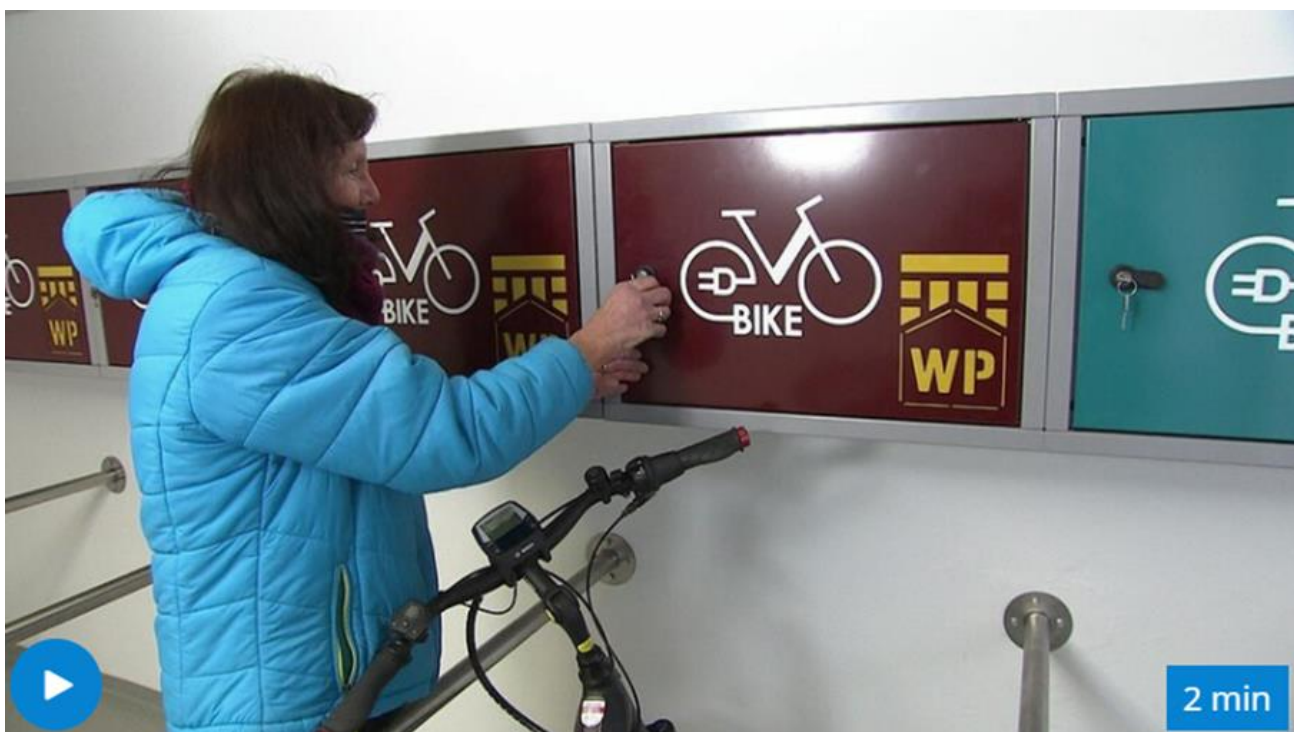
E-bike charging station in Triptis, Thuringia, Germany, provided to its tenants by the public housing company. 13
