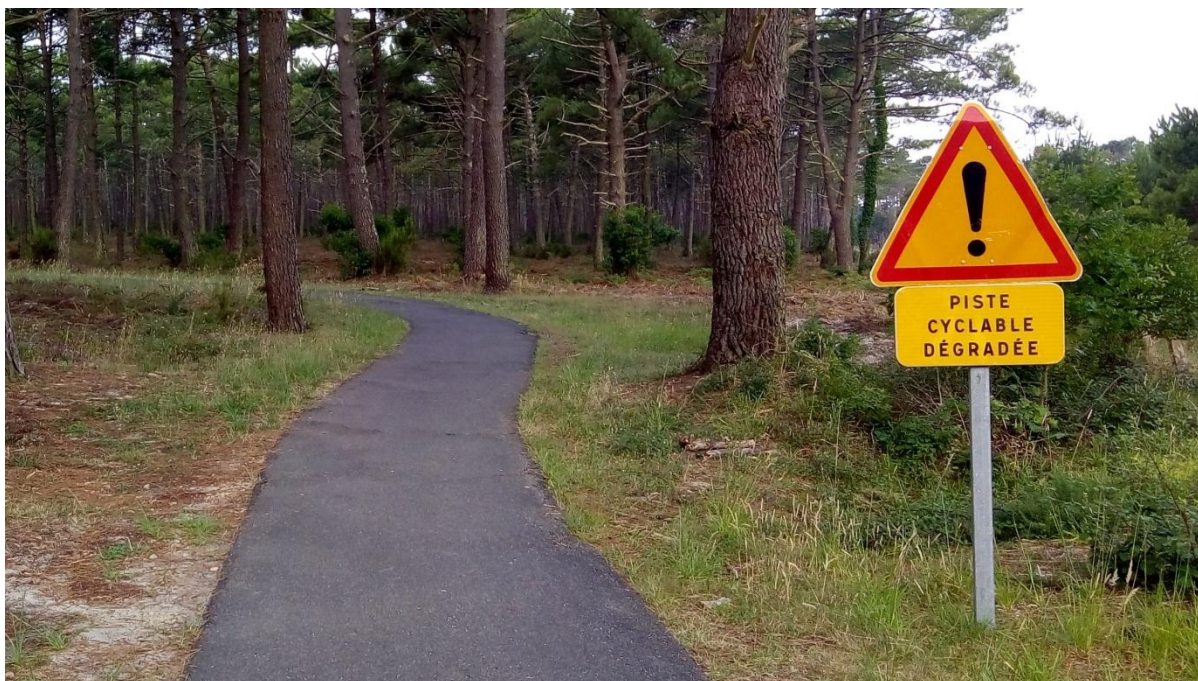
Figure 31. Root-related damaged on EuroVelo 1 in France.
