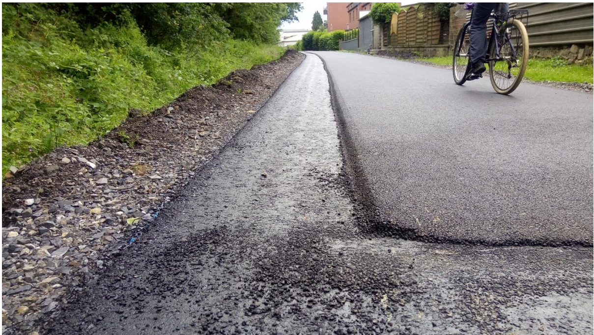
Figure 8. Layers of asphalt surface under construction. The base layer is wider to accommodate a gravel shoulder for horse riding without risking damage to the construction of the cycle track. EuroVelo 3, Belgium.
