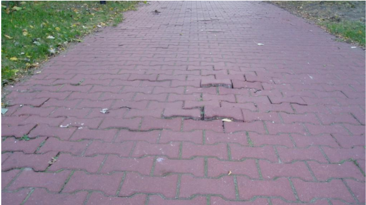
Figure 16. Damages on paving blocks surface a few years after opening. Warsaw, Poland.
