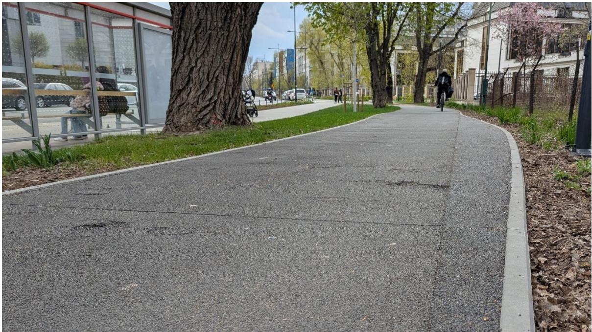
Figure 28. Damages to resin-bound surface one year after opening. Jana Kazimierza street, Warsaw, Poland. Photo credit: Marek Smyk.
