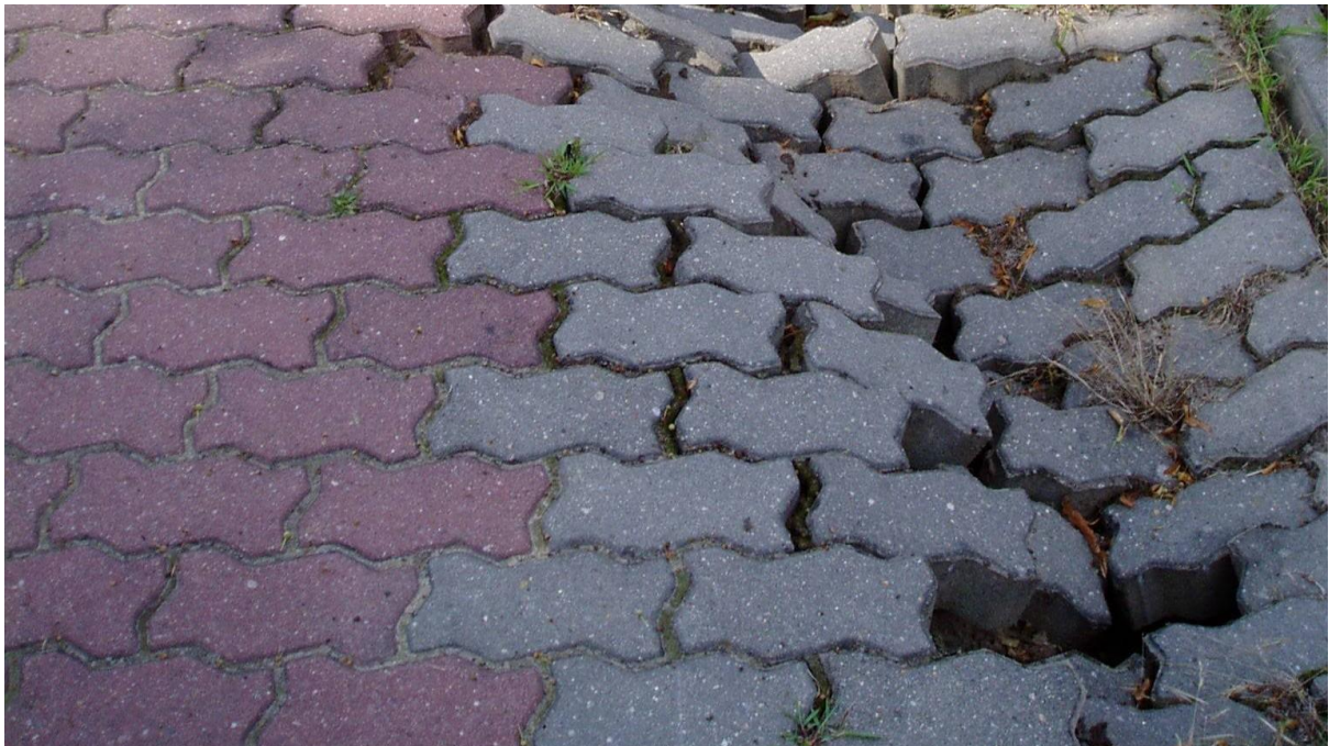
Figure 17. Water seeping in between paving stones rinses out the underlying base layer. Frankfurt an der Oder, Germany.
