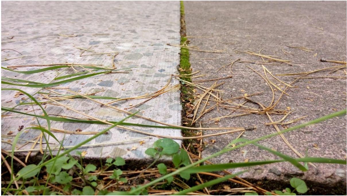
Figure 11. Concrete plates move with time, which increases the gaps and creates a height difference between the plates. The concrete plate on the left has been ground (sanded?) to alleviate the difference in height. Near Lommel, Belgium.
