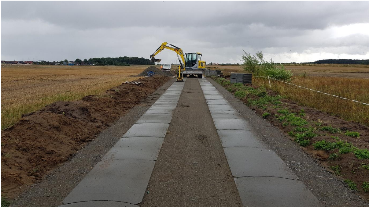
Figure 13. Concrete lanes (each 80 cm wide) built with interlocking plates with articulated joints. Szczecin Lagoon Cycle Route, West Pomerania, Poland. Photo credit: Wanda Nowotarska.
