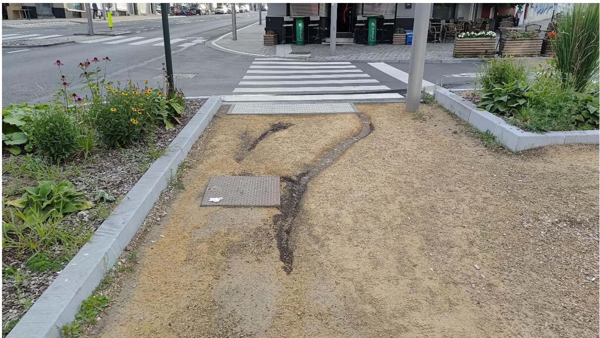
Figure 23. Gravel surface damaged by rainfall. Brussels, Belgium.
