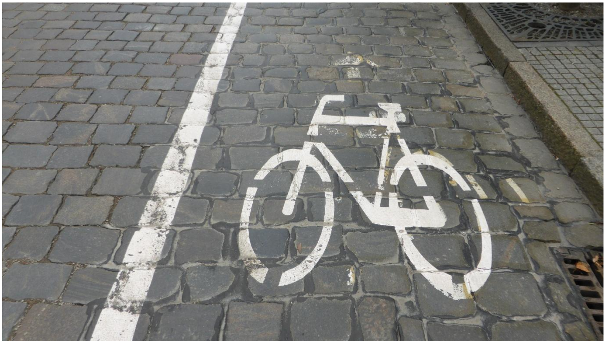
Figure 20. Filled gaps in between stone blocks on a cycle lane only. Klaipeda, Lithuania.
