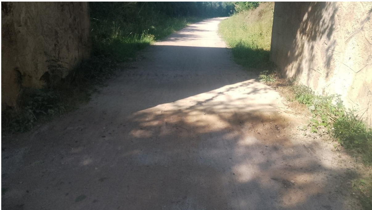
Figure 25. Potholes in gravel surface created by water dripping from the bridge above. V819 cycle route (Chemin des Droits de l'Homme) between Castres and Albi, France.
