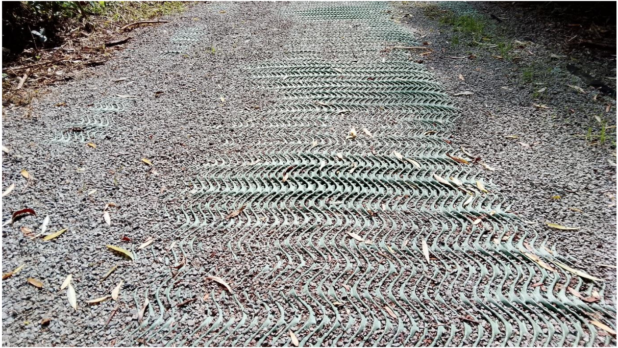
Figure 29. Deteriorating permeable gravel surface. Near Enghien, Belgium.
