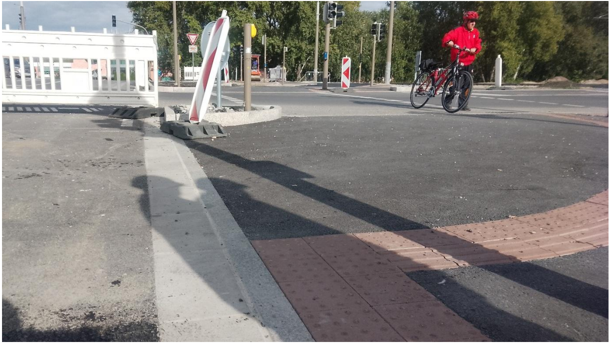
Figure 36. Dropped but still protruding kerb on a new cycle crossing. Bratislava, Slovakia.
